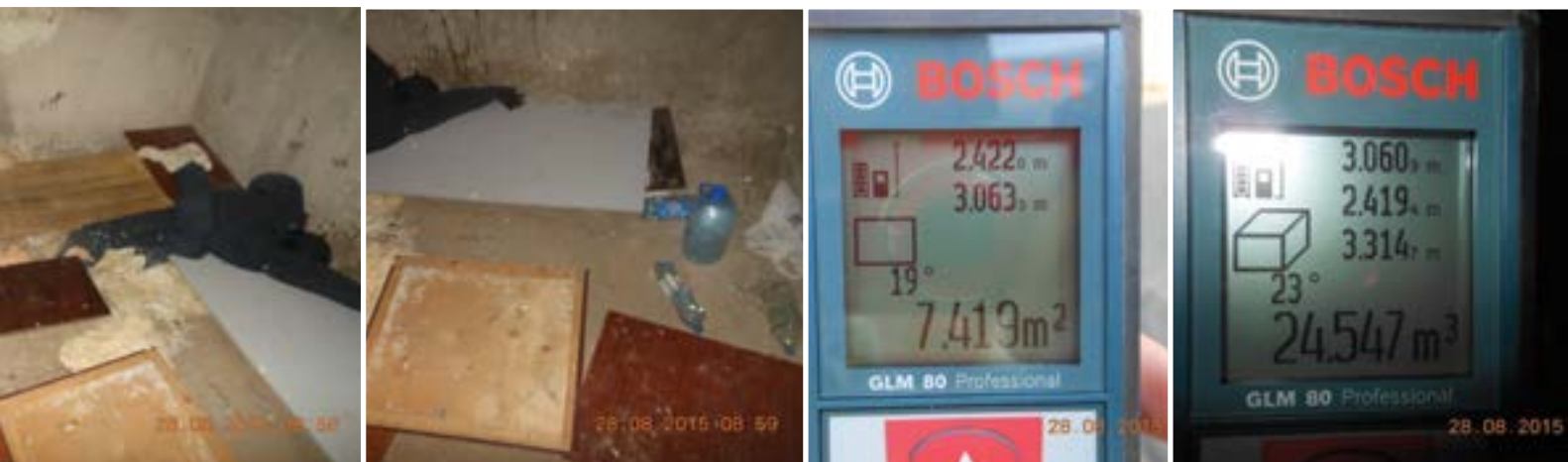
Photos 29-32. Conditions of detention at the basement of the State scientific research and design institute of nitrogen industry and organic synthesis products in Syevyerodonetsk.
