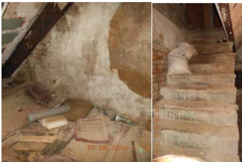
Photos 1-2. Basement of Kostyantynivka city council (Donetsk region, Kostyantynivka town, 260 Lenina str.).
